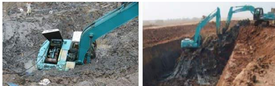
Figure 17. Pre-vacuum: excavator sank into soft clay, post vacuum: trenches were excavated with ease (courtesy of PT. Geotekindo)
